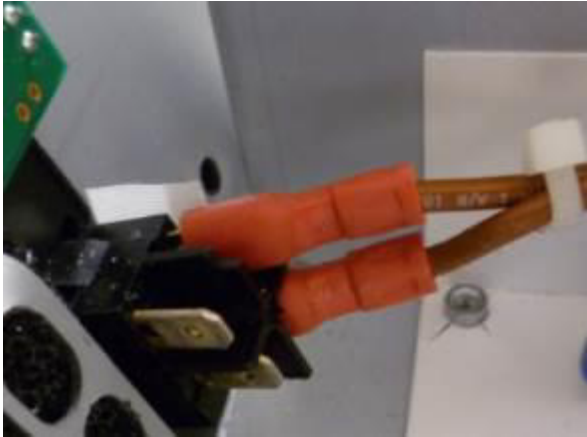
Wiring to mains switch
