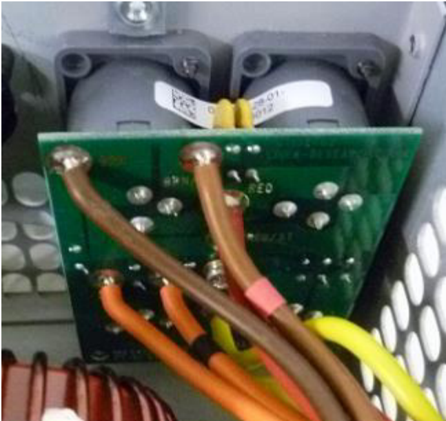
Wiring at rear of speaker connectors
