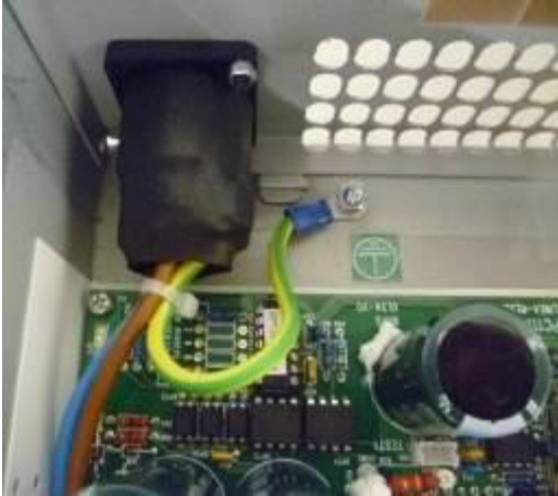
Mains inlet and earth wiring
