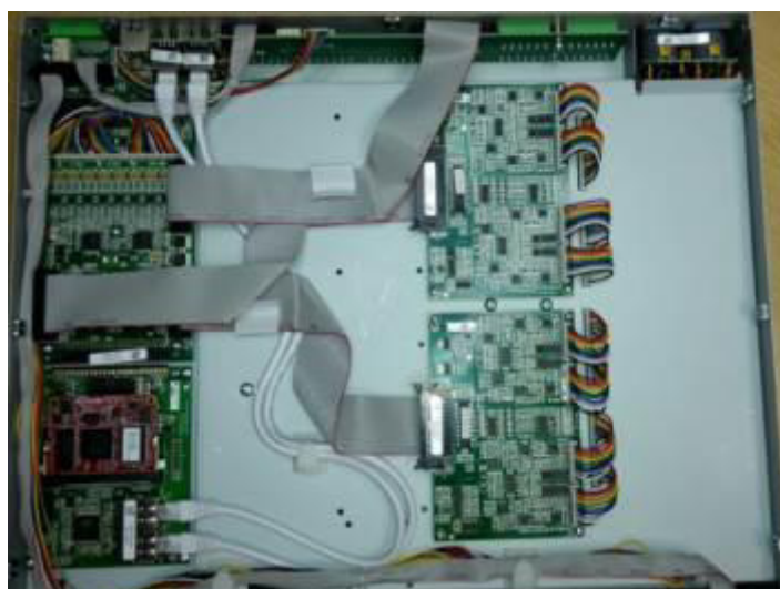
8 channel with Dante card fitted
